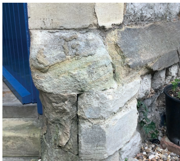
m. Erosion of stonework at low level adjacent to turret door.
