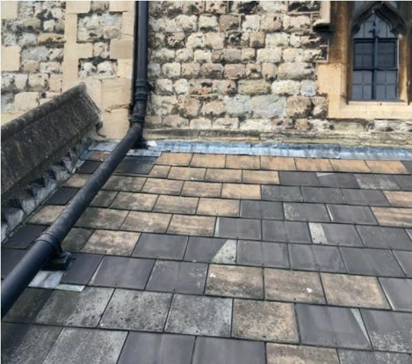
U. West end showing RWP from nave roof crossing aisle roof and slipped/damaged slates.
