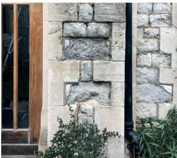
l. Typical erosion of Kentish Ragstone at buttresses.
