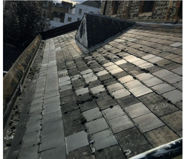
V. View looking west showing defective flashings at parapet and redundant dormer.
