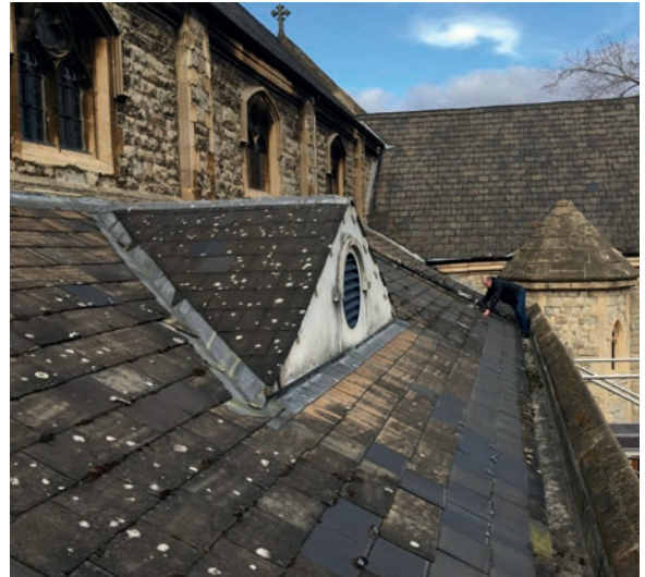
X. View looking east showing existing asphalt gutter and replacement fibre cement slates at low level.
