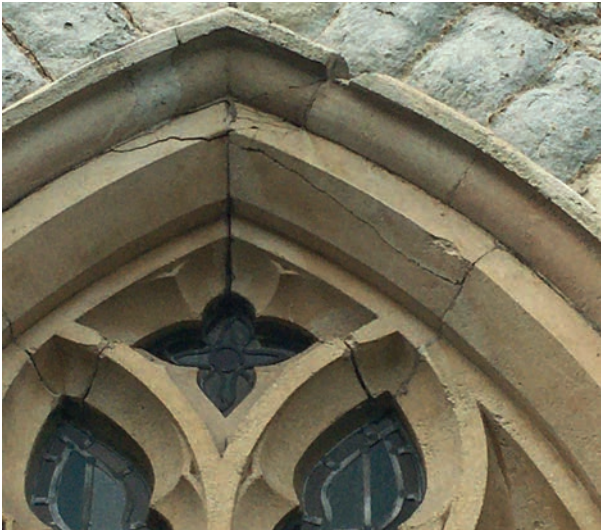
q. Cracking across stonework to window surround - south aisle.
