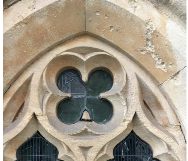
b. Fractured stonework at quatrefoil window - east elevation of south porch.
