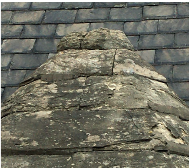
s. Erosion of turret roof apex stone.
