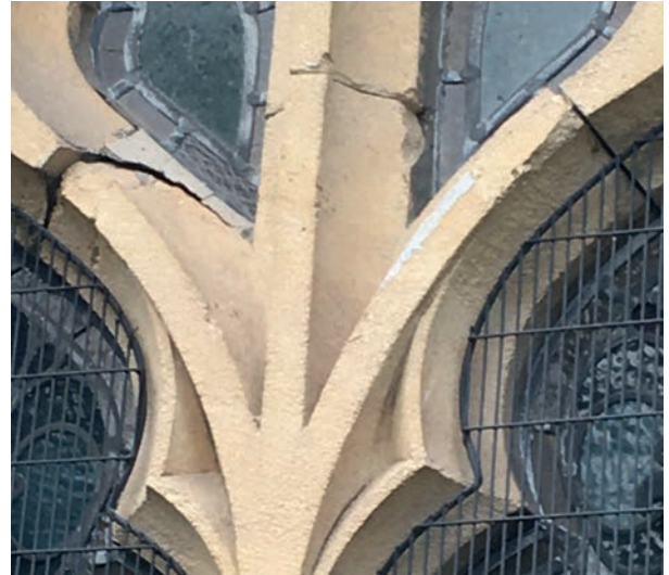
p. Previous mortar repairs to tracery - south aisle.
