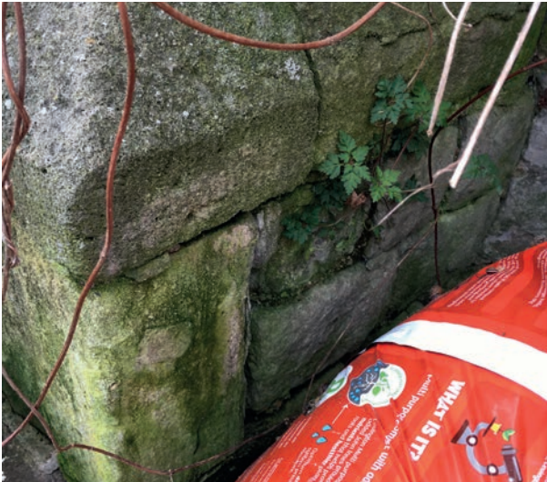
c. Typical deterioration of stonework at plinth.
