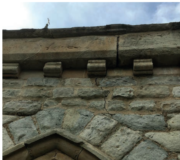
k. Typical cracking through parapet stonework above south aisle window heads.
