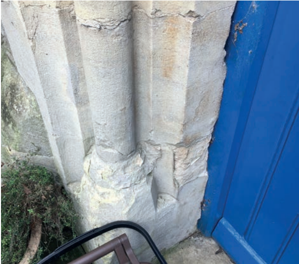
a. Erosion of stonework at low level - south porch.
