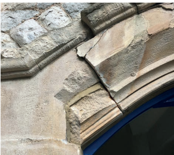
e. Erosion of hood moulding and fractures to stonework at turret door head.
