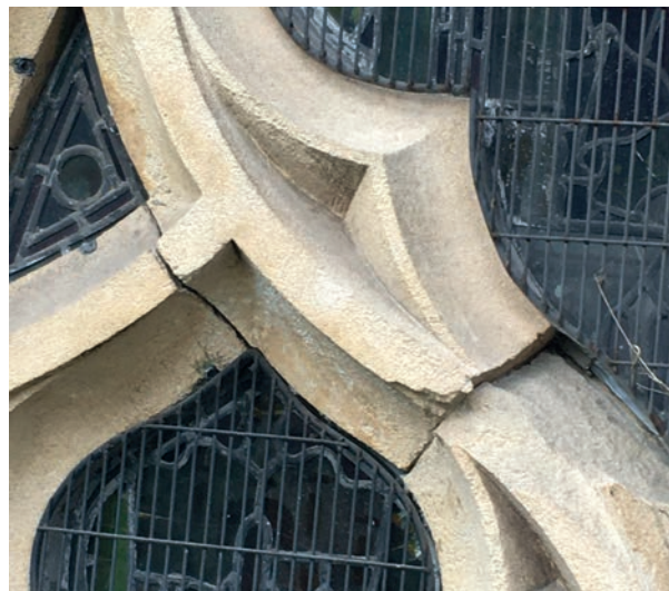
h. Fractures through south aisle tracery.
