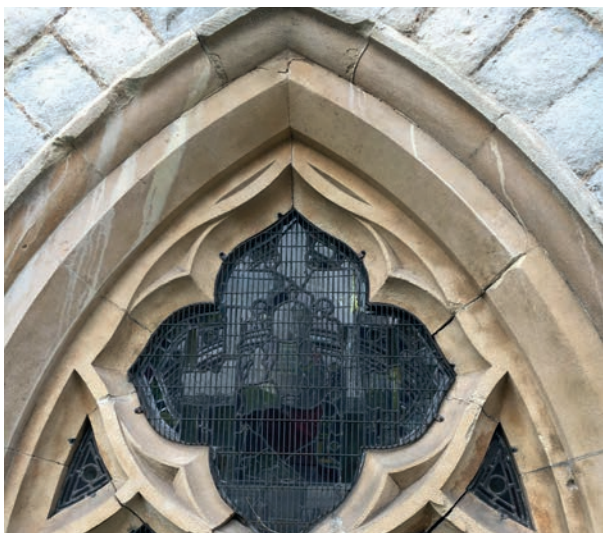
j. Open joints and eroded hood moulding - south aisle window surround.
