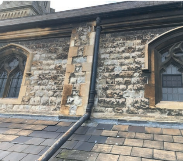
W. Patches of defective slates with more recent patch repairs in fibre cement.
