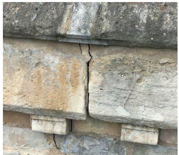
t. Open joints to turret roof corbel.
