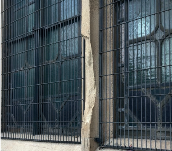
n. Spalled stonework to window mullion - south aisle.
