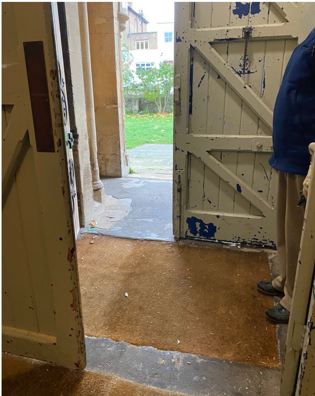
Figure 5: Main church door leads to several uneven changes of level, which could be marked with yellow strips. Both doors need to be opened for a wheelchair to pass through.
