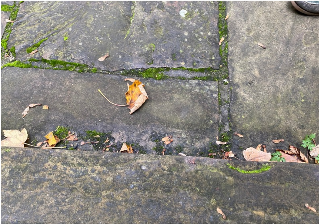
Figure 4: Some paving stones are uneven on path leading to the church entrance
